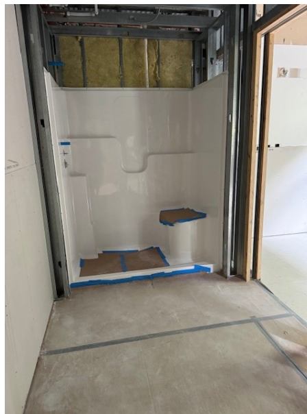
Part of he bathroom showing shower installed.
