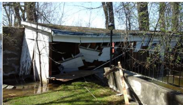
The condition of the white cabins after the flood
